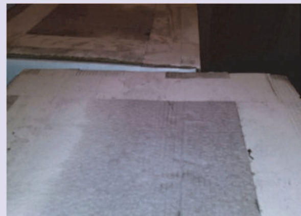
Unstable floors covered in cardboard
