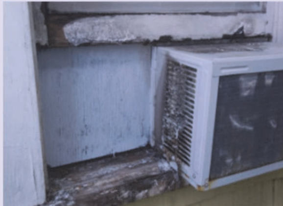
A moldy air conditioner and rotten window frame
