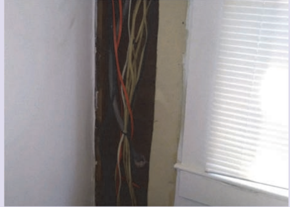
Exposed electrical wires
