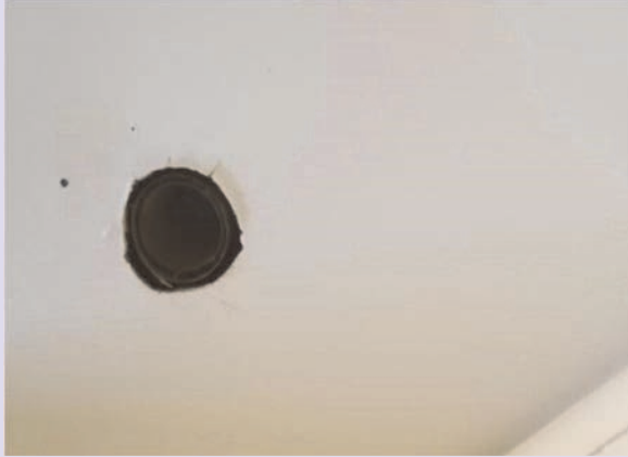
Water drained onto the kitchen floor through this open hole in the ceiling.
