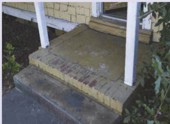
The front entrance to the home was not accessible or ADA compliant.
